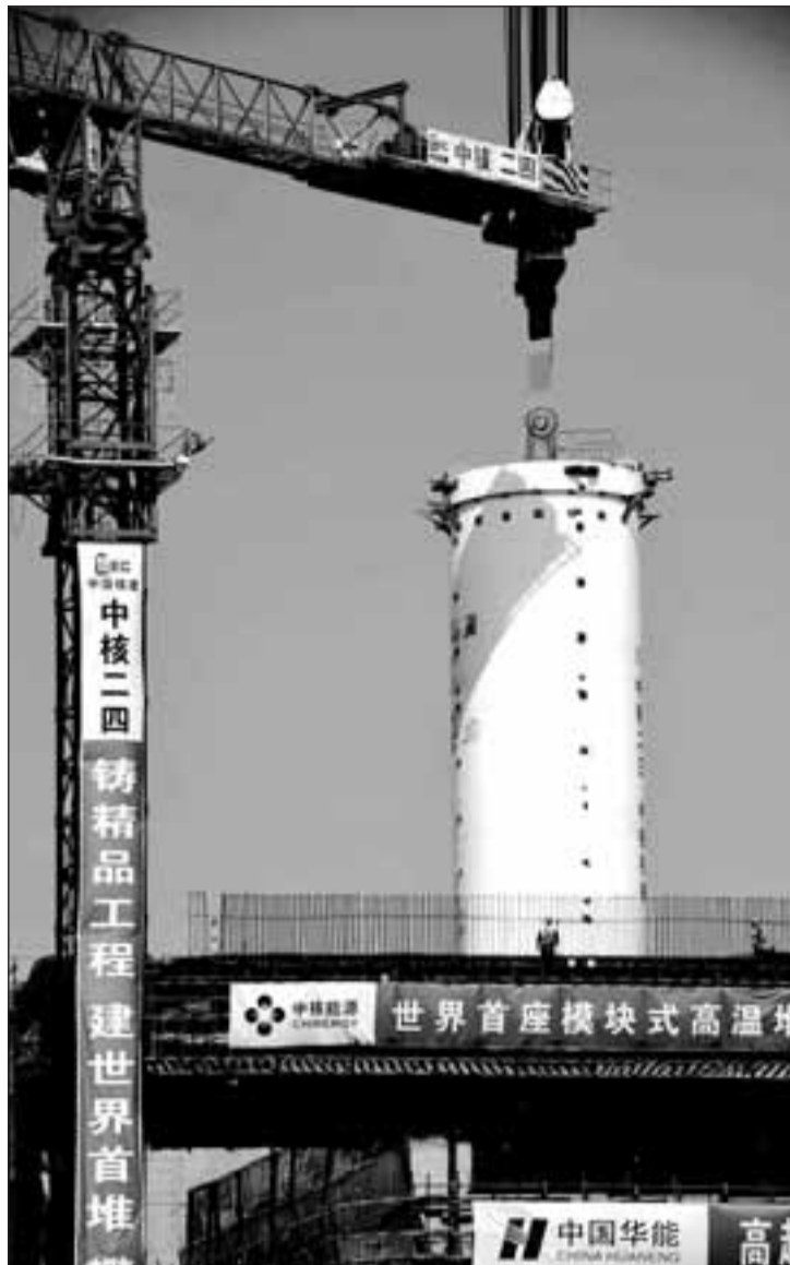
A crane lifts a key component of China's first fourth-generation nuclear energy system before installing it in Huaneng Shidao Bay nuclear power plant in Shandong Province. — Xinhua
